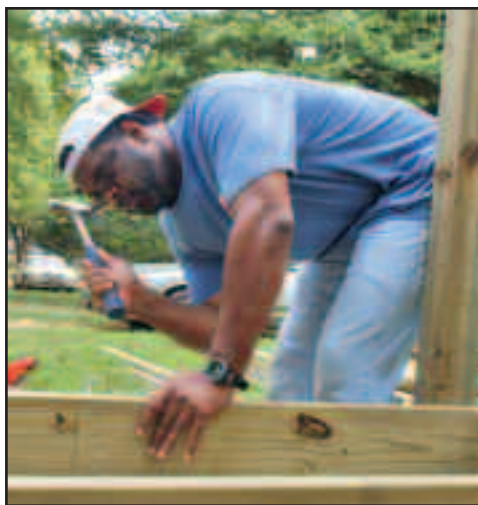
Ralph Carmouche, director of food services at Baptist Women's Hospital, builds a wheelchair ramp during the United Way Day of Caring. Construction skills and help of all kinds will soon be needed, as Baptist plans to begin construction on a home for Habitat for Humanity.
